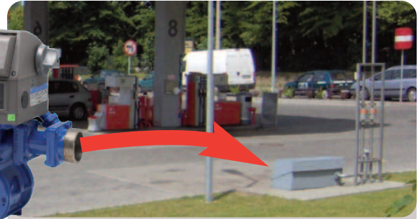
Connection to underground tank
